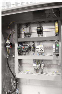
View inside electrical panel.
